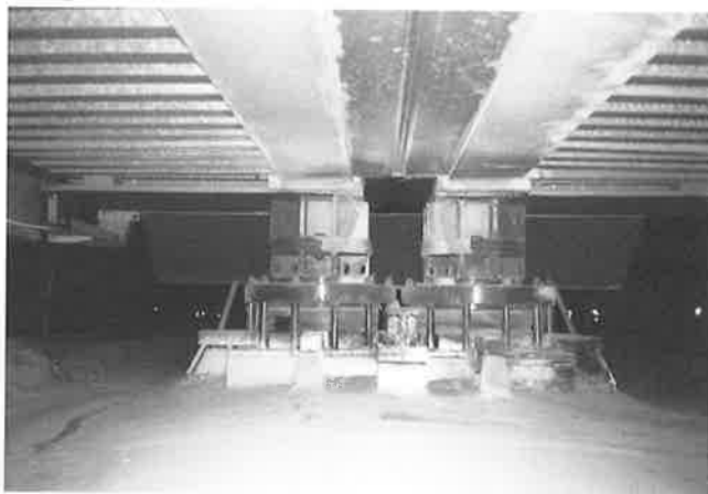
写真-3-1 積層ゴム支承
