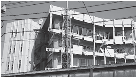
Figure 6. Damage to Uto City Hall
