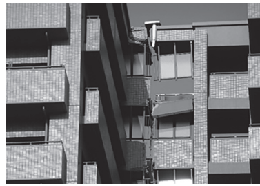
Figure 7. Damage to expansion joints
