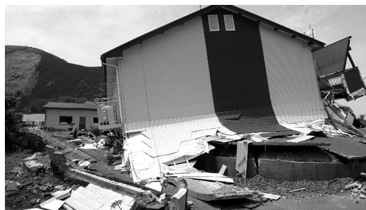
Figure 5. Damaged wooden apartment in Minamiaso Village
